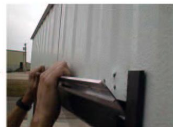
Figure 8 (viewed from interior)
